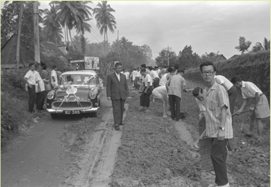
Members of Serangoon Gardens Citizens’ Consultative Committee, residents of Cheng San Road and members of vigilante corps, led by Member of Parliament for Serangoon Gardens R A Gonzales, repairing a mile-long stretch of Cheng San Road, off Serangoon Garden Way, damaged by floods, 1967.
